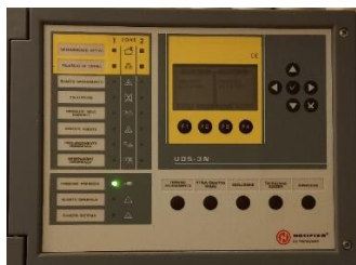
"NOTIFIER AM-2000" LOCALE DISASTER RECOVERY
